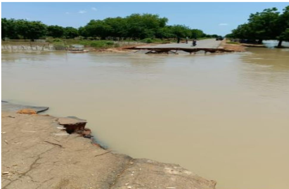
Figure 2. Flood destroyed a major highway in Northern Nigeria
