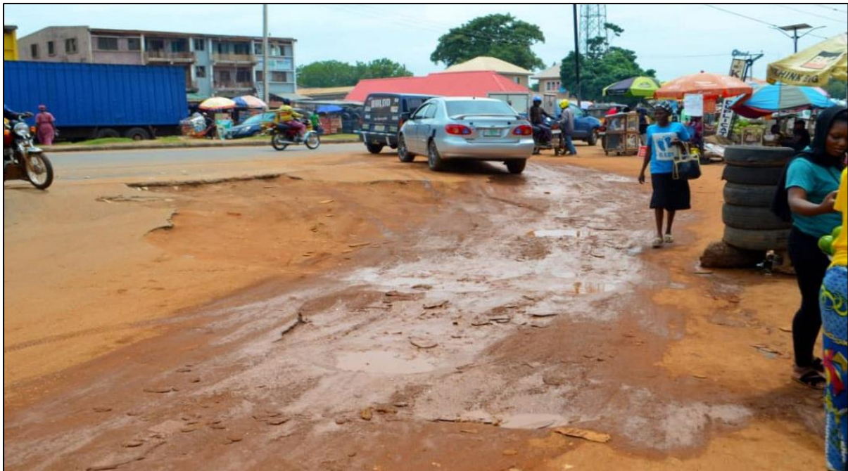
Plate 1: Poor Condition of Road Pavement at Kilanko-Offa Garage Road, Ilorin Source: Field Survey, 2024
