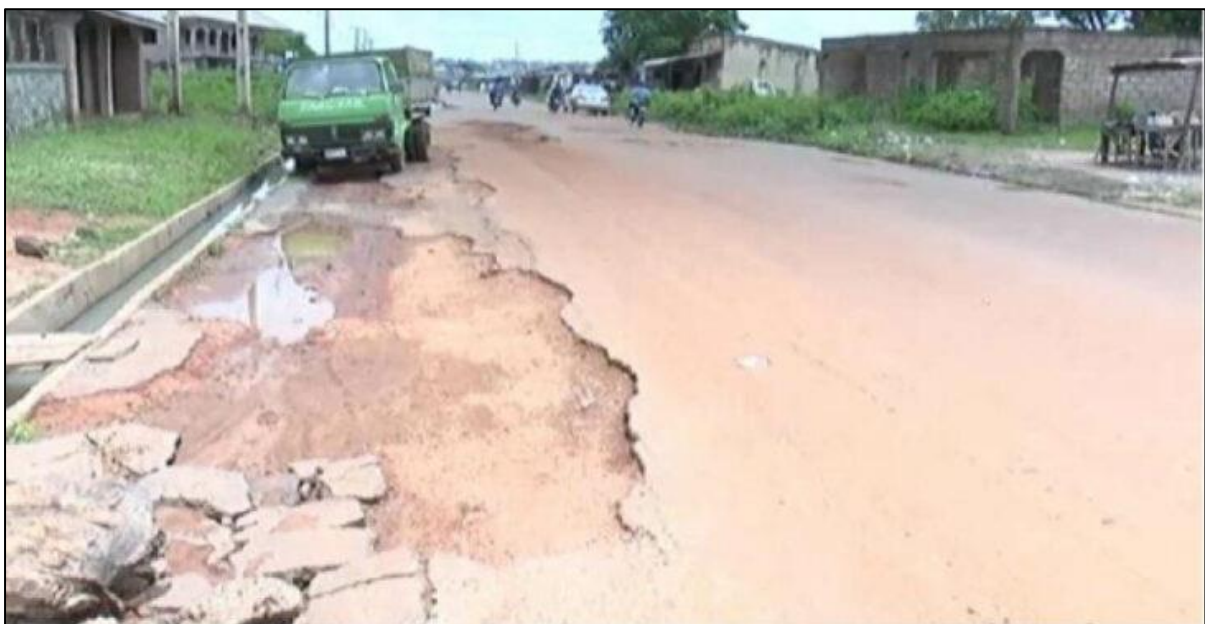
Plate 2: Poor Condition of Road Pavement at GRA, Ilorin Source: Field Survey, 2024
